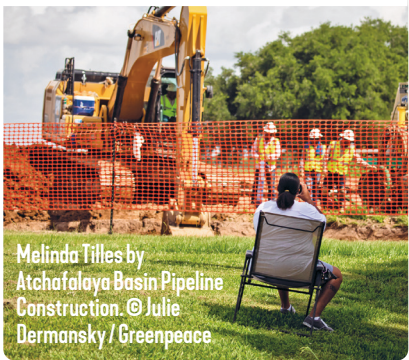
31 March 2018, Acadia Parish, Louisiana. Construction on the Bayou Bridge Pipeline. © Julie Dermansky / Greenpeace
