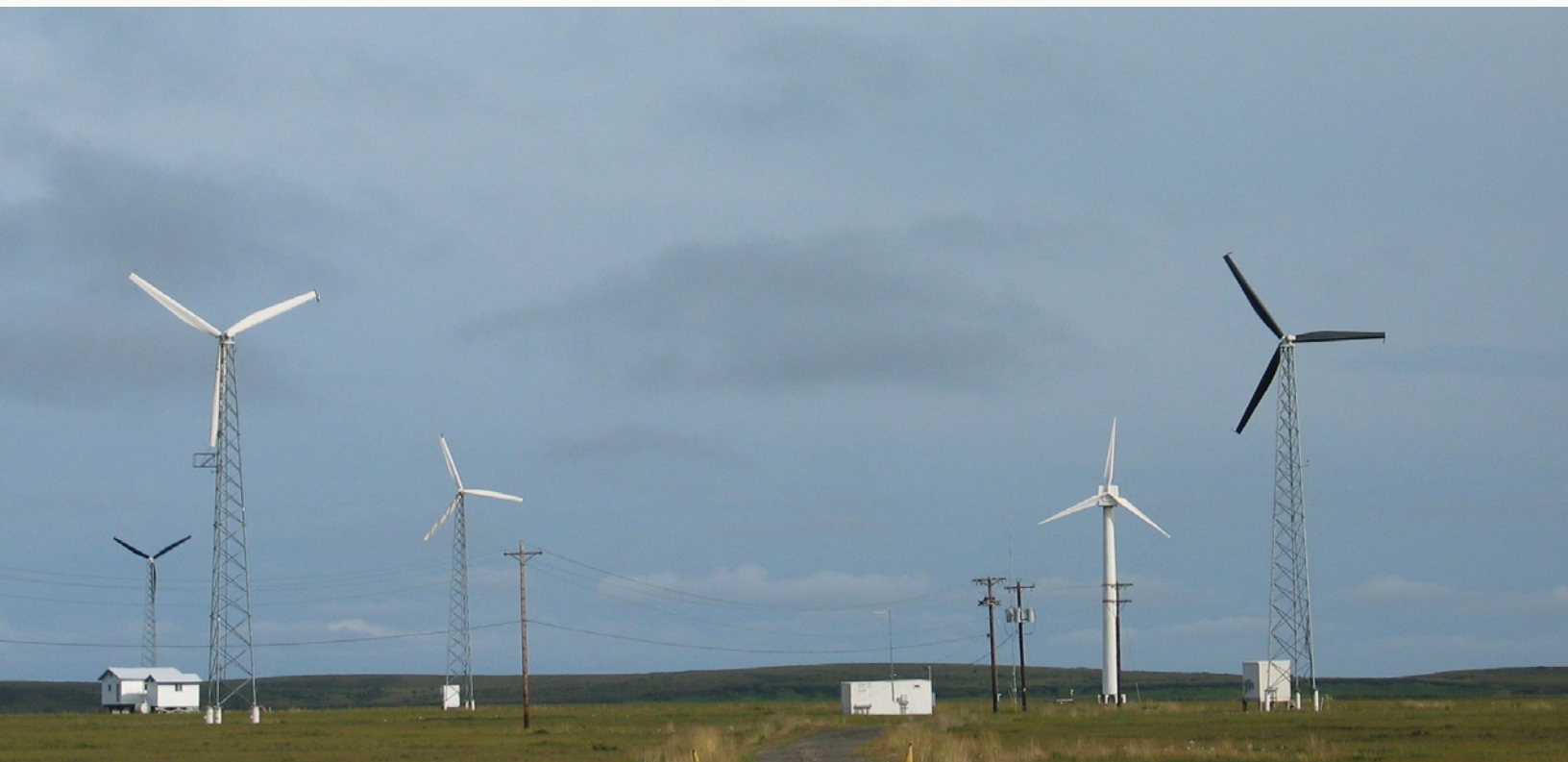
Seventeen wind turbines provide up to 1.14MW of electrical capacity to Kotzebue, reducing reliance on costly diesel fuel. (Wikimedia Commons)
