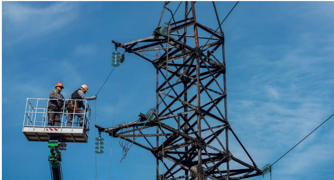
Figure 8. A photo of a crew repairing electricity grids in Ukraine after a Russian missile attack has damaged the infrastructure. Author: unknown; Source: DTEK
