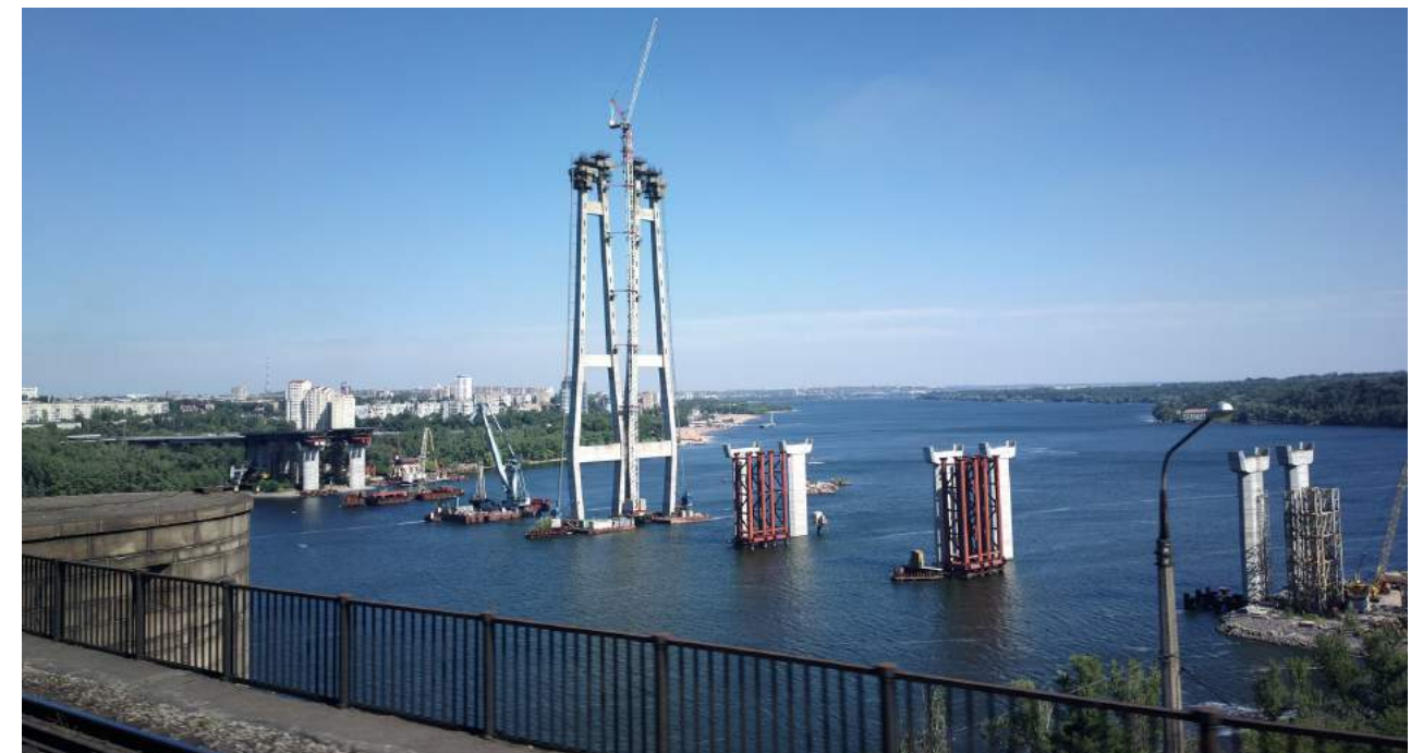
Figure 16: Photo of the construction of the New Bridge across the Dnipro and Old Dnipro in Zaporizhzhia, 2015 Author: Teteria Sonnna ; Source: Wikipedia (CC BY-SA 2.0)
