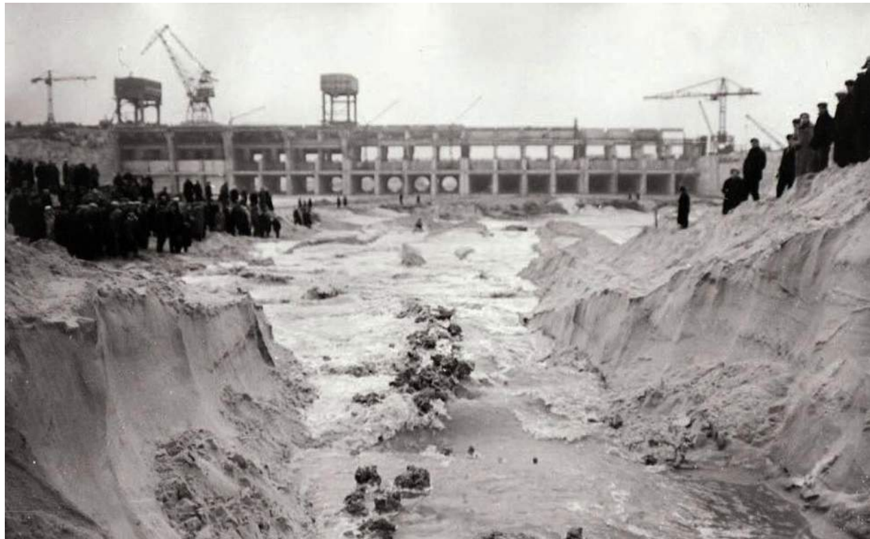
Figure 14. Photo from the construction of the dam for the Kyiv HES (early 1960s). Author: unknown. Source: Ukrhydroenergo
