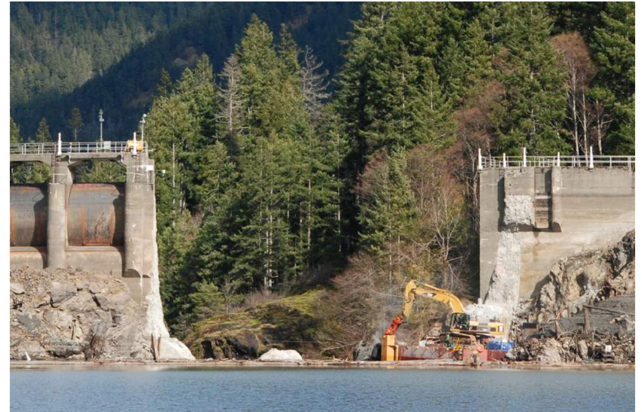
Figure 6. Photo of the Glines Canyon Dam, the largest dam ever to be removed, shown mid-demolition in 2012. Author: Olympic National Park; Source: Wikipedia.org (Public Domain) – Photo chosen for illustrative purpose
