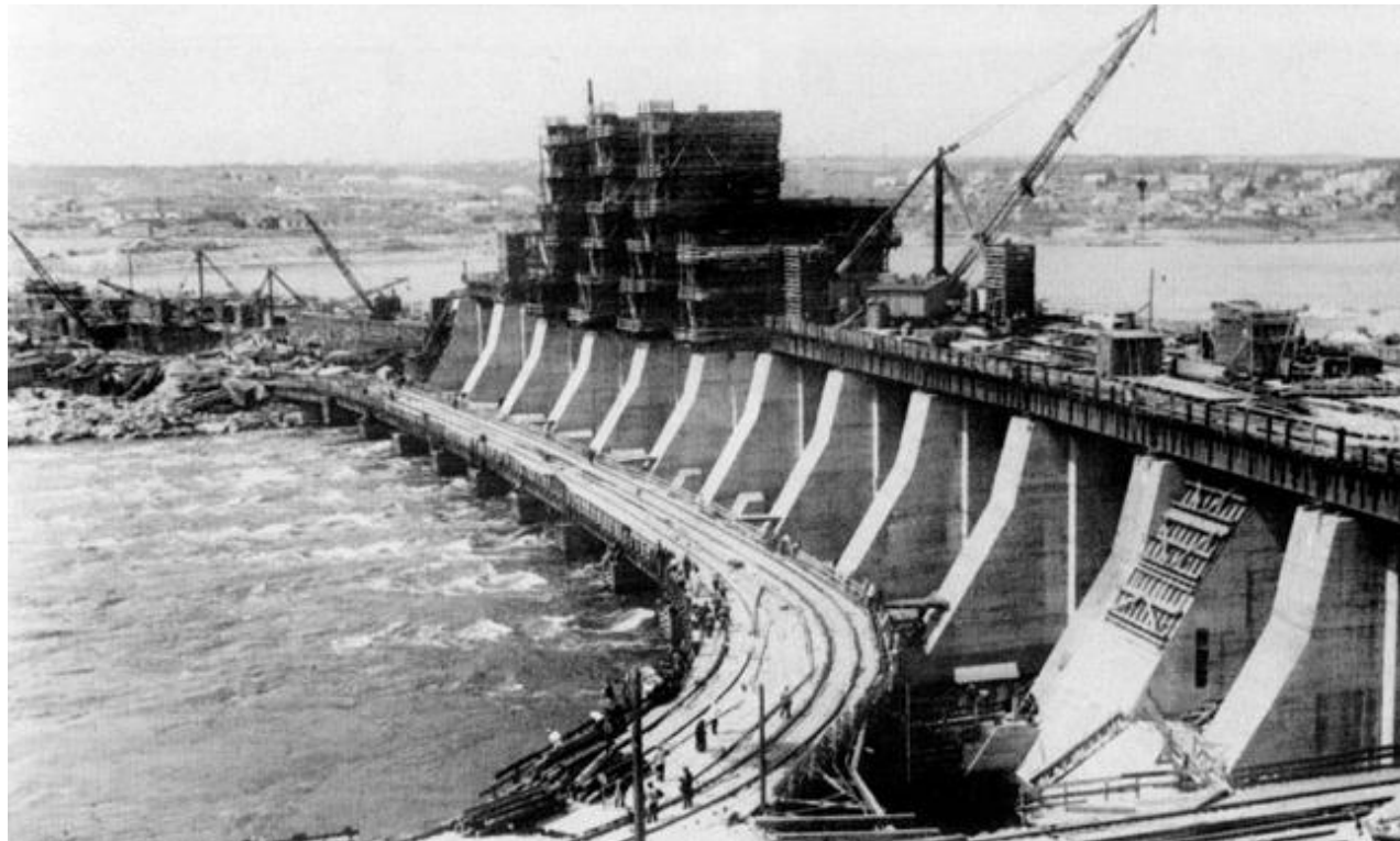
Figure 11. Photo of the DniproHES under construction, 1934 Author: unknown; Source: Wikipedia.org (Public Domain)
