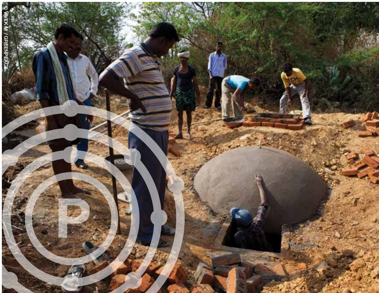
Image Workers building a new biogas unit in Kammavaripalli, Bagepalli taluk, India.
