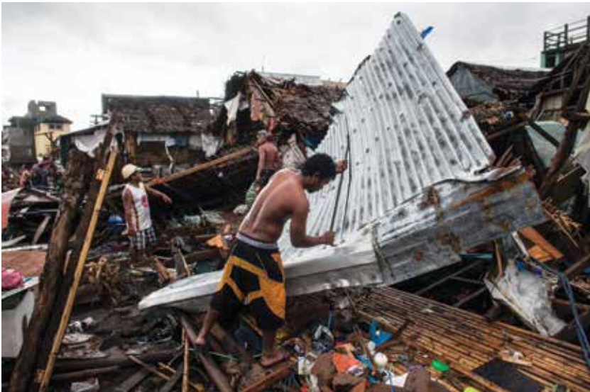
Workers repair damaged buildings in the aftermath of Typhoon Kammuri in Legazpi City, in the province of Albay, Philippines.
