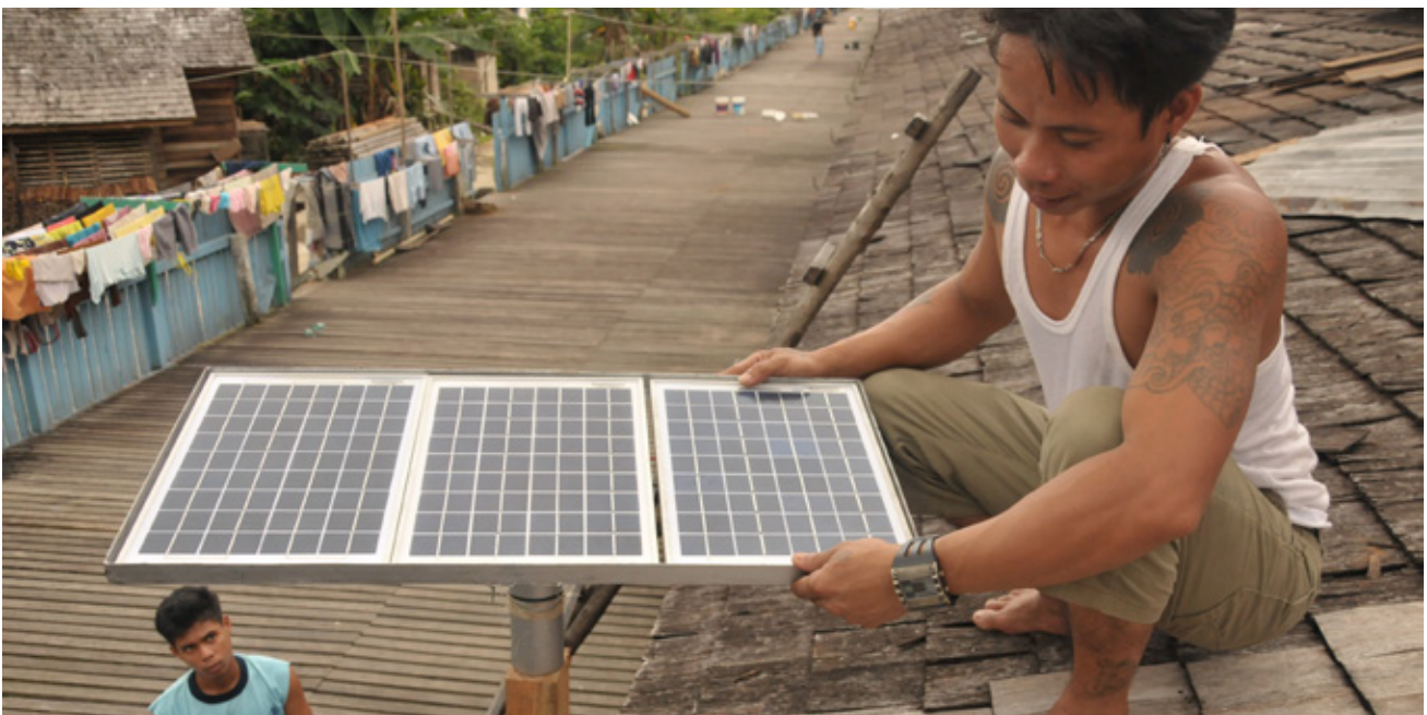
© Enter Indonesia / Greenpeace. Installing solar panels on the communal longhouse. The area where the people of Sungai Utik live does not have access to electricity.
