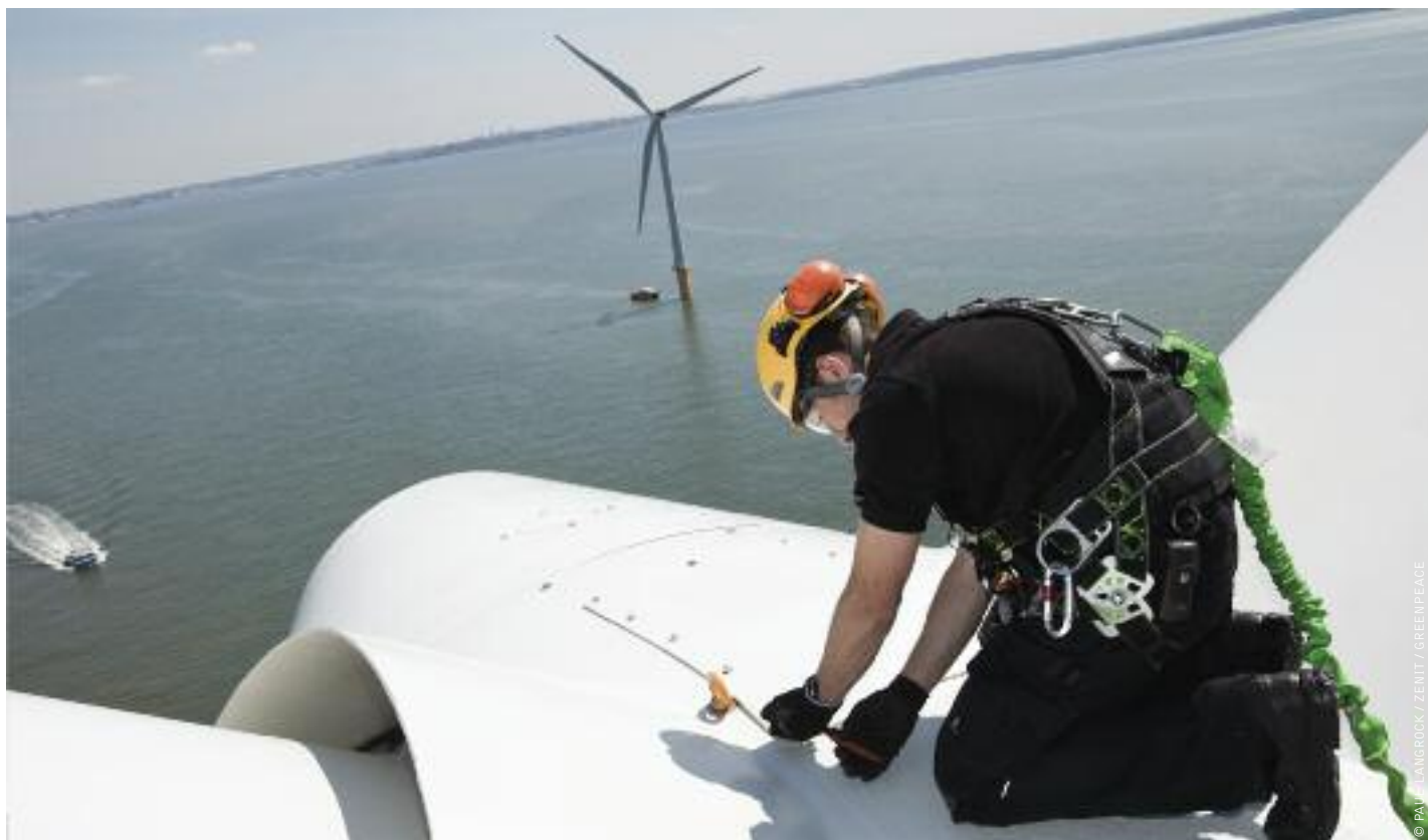
image BURBO BANK OFFSHORE WINDPARK 7 KILOMETERS OFF CROSBY BEACH. TECHNICIAN DAN SIMMONS WORKING ON TOP OF A WINDMILL. THE 25 WIND TURBINES OF TYPE SIEMENS SWT 3.6 107 A 3.6 MEGAWATT AND ARE OPERATED BY DONG ENERGY.
