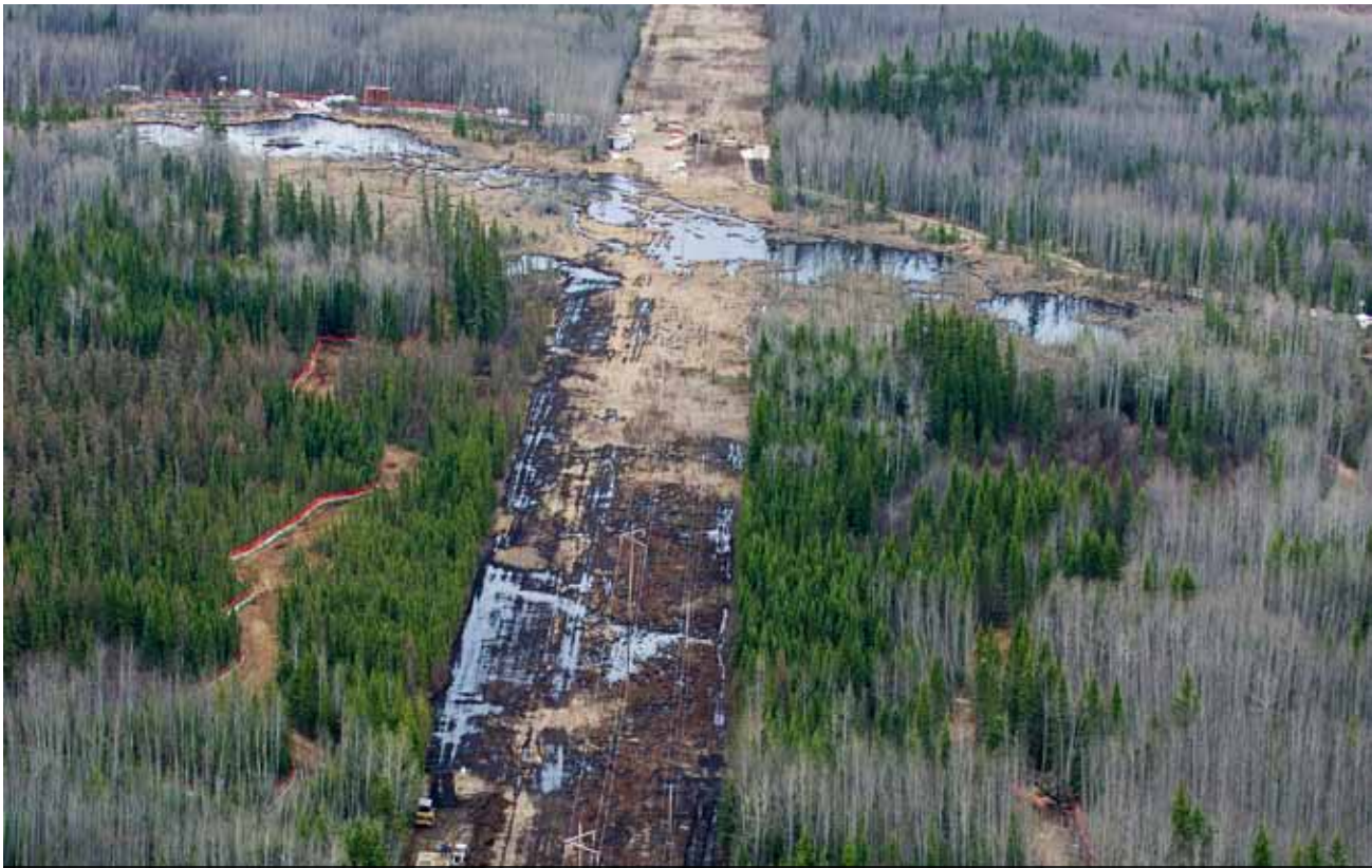
A view of the clean up operations at the Rainbow Pipeline oil spill.
