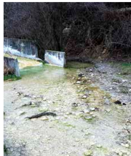
Figure 7. The concrete channel leading out of the LEF along the Kamenishka river
