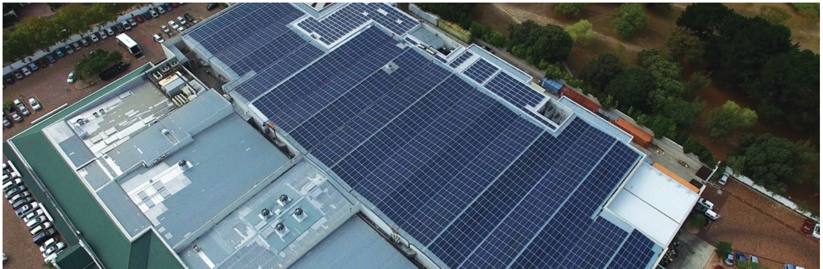
© Growthpoint Property. Constantia Village Solar PV Installation, 2016.
