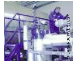
image FIRST GEOTHERMAL POWER STATION IN GERMANY PRODUCING ELECTRICITY. WORKER IN THE FILTRATION ROOM.
