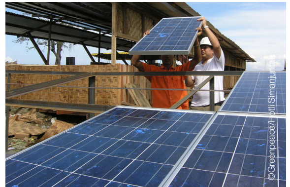
Greenpeace donates a solar power system to a coastal village in Aceh, Indonesia.
