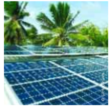
image SOLAR PANELS ON REFRIGERATION PLANT (FOR KEEPING FISH FRESH). LIKIEP ATOLL, MARSHALL ISLANDS.
